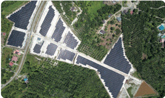
13MW, Malaysia Beaufort Solar cable
