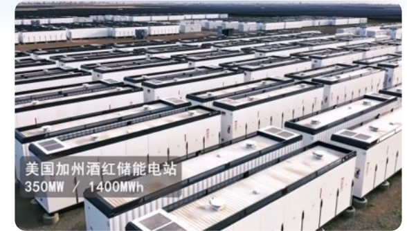
350MW, USA Crimson Energy storage cable & Connector
