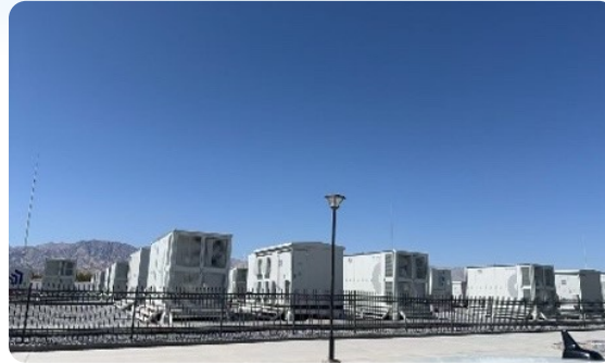
800MW, China Qingdao Energy storage cable & Connector
