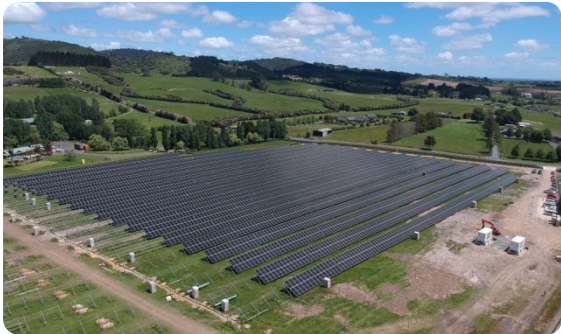
7.6MW, South Auckland DC Solar cable
