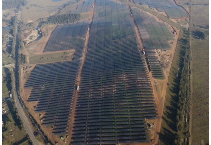
System capacity: 95.2MW Chile
