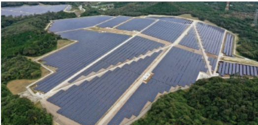
System capacity: 50MW Japan
