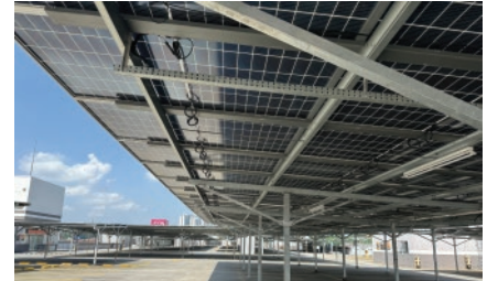
System capacity: 3MW AEON carport, Malaysia
