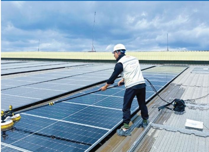
PV Module Cleaning
